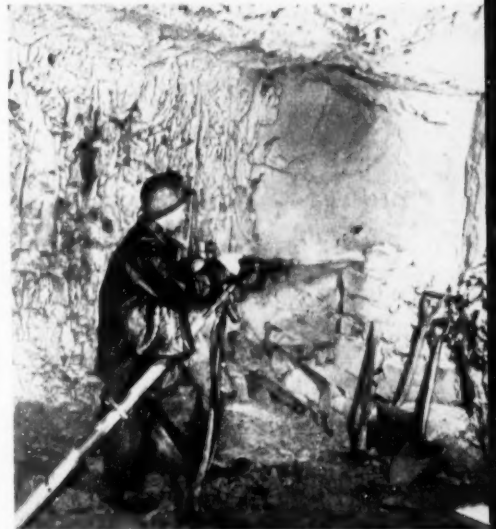
An air leg, mounted jackhammer is used to drill a drift round. Note the frost incrustated face and back.
